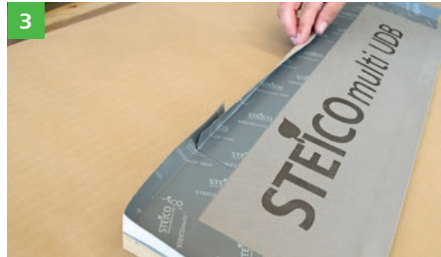
The STEICOmulti tape F adhesive strips are then attached to the insulation wedge in such a way that a three-sided „trough“ is formed.
